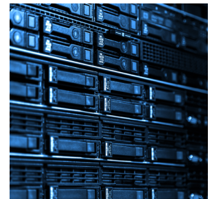
Data Center Servers
